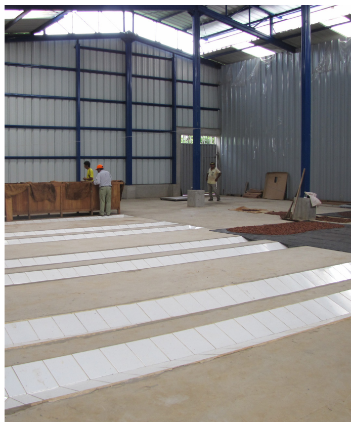
New processing plant for fermentation, drying and storage of cocoa.
