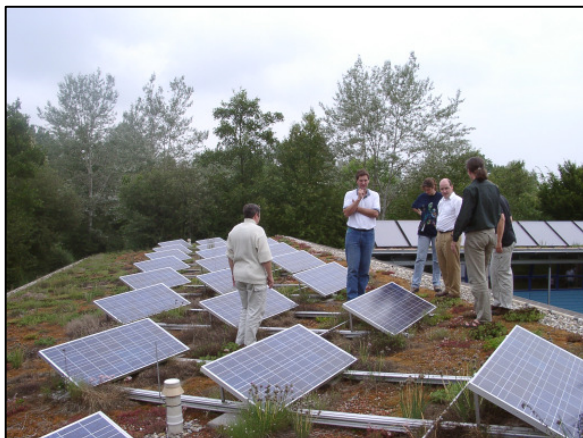
Solar Technology at Camp Grounds – ECOCAMPING at Lake Constance Photo: GNF
